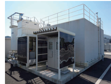
Our in-house wastewater treatment facilities
