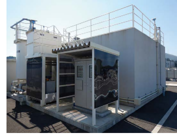
Our in-house wastewater treatment facilities
